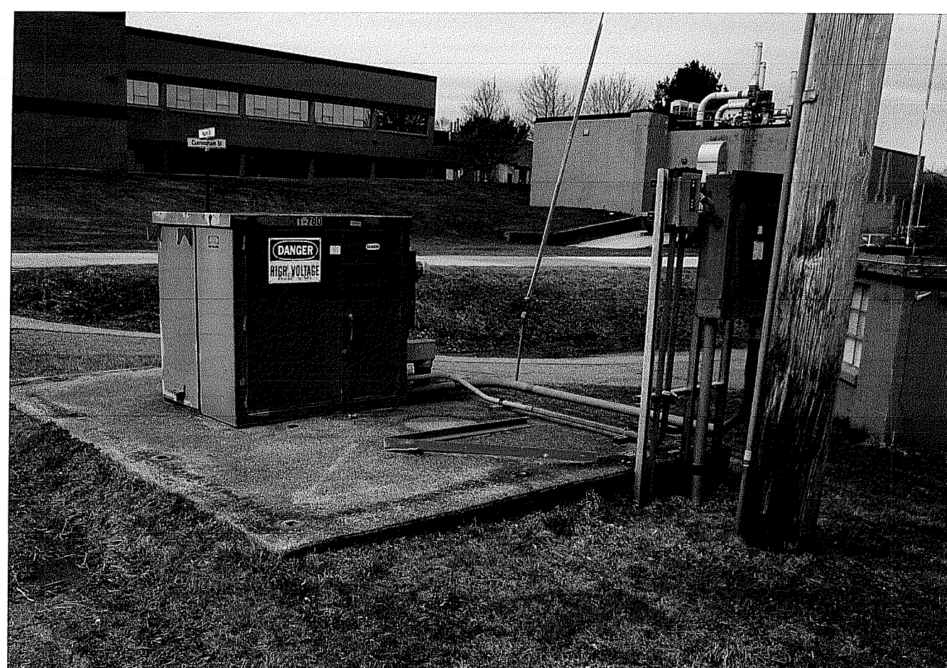
PHOTO AT EX. XFMR T-780
